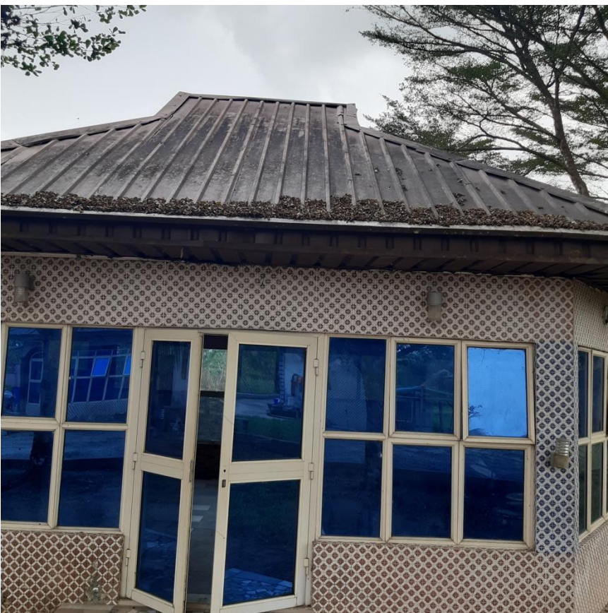
Figure 8: The leaf litters also affects the roofing sheet
