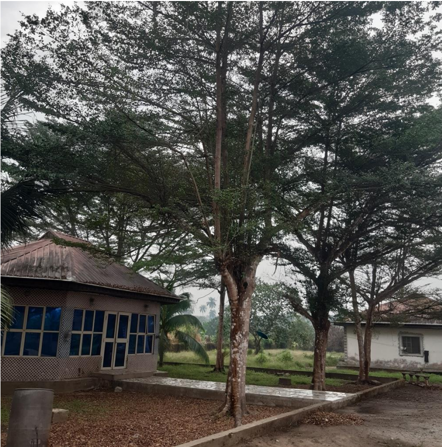
Figure 7: Leaf litters on the roofing sheet
