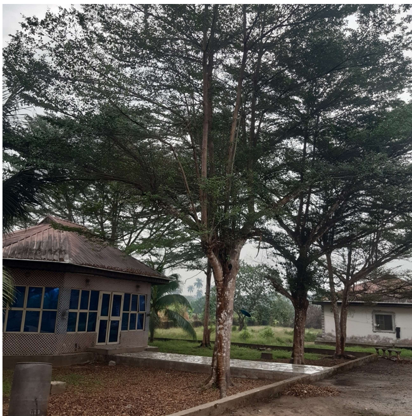
Figure 7: Leaf litters on the roofing sheet
