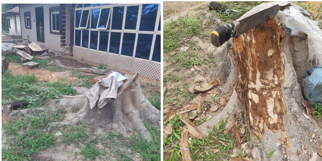
Figure 3: This tree with buttress root have been cut down because of the damages being caused to the foundation of the nearby building
